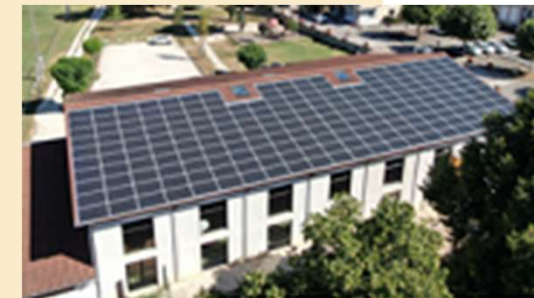
Vourey - Gymnase 84kWc
